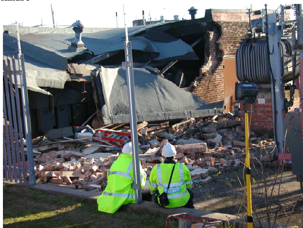
Figure 1 Damage to substation following a catastrophic switchgear failure
